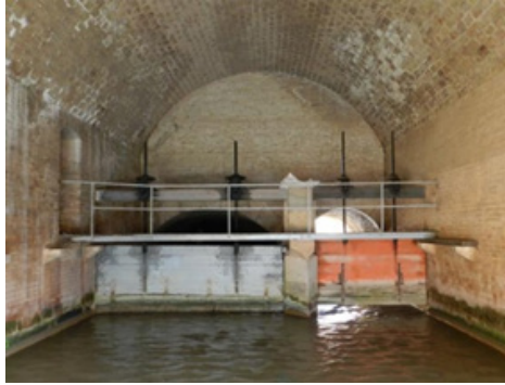
Figure 5: Hydraulic Infrastructure Elaborated by the authors.
